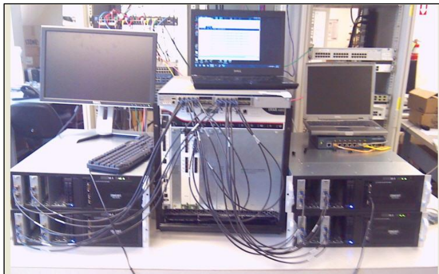
Four-node cluster. Shown above is the multi-node configuration. Two McAfee NGFW 5206s are on the left and two are on the right. The BreakingPoint test system sits between them. Atop the BreakingPoint is the Cisco 4500X switch.
